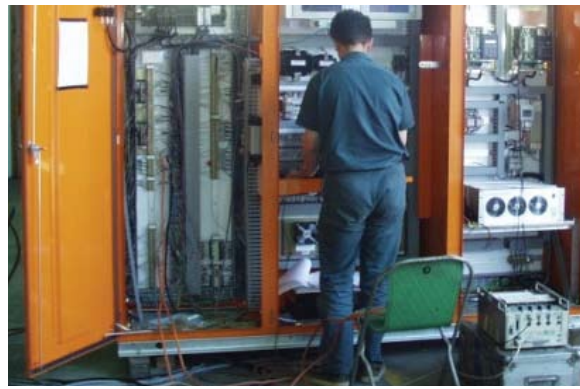
Electrical Control Cubicle
